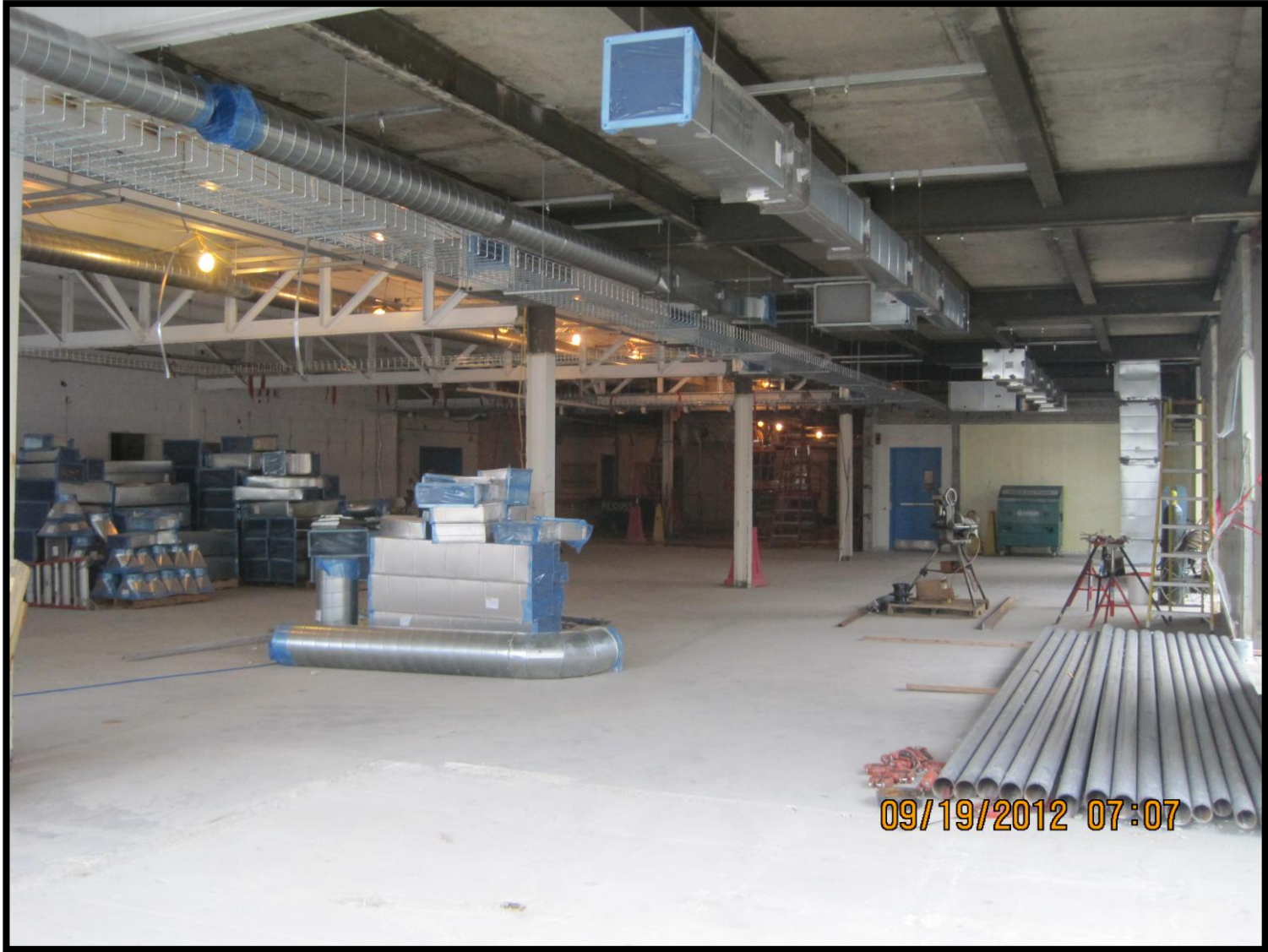
Test Lab New HVAC duct
